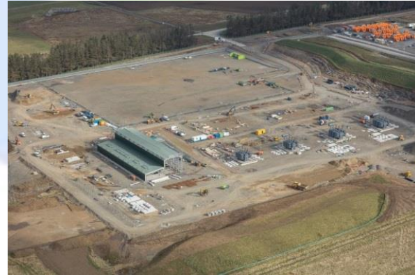
Photograph of the Spittal 275kv/132kv AC Substation in the foreground under construction, the 800MW HVDC Converter site area in the background and the HVDC cable drums in the site compound to the right hand side.
