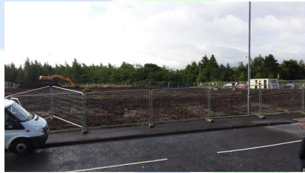
The National HVDC Centre , site photograph, June 2016
