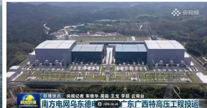
Wudongde–Kunliulong HVDC China transmission project commissions Hybrid converter elements.
