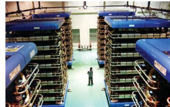
India's Sassaram BtB upgrades LCC->VSC, 0.5->1GW.
