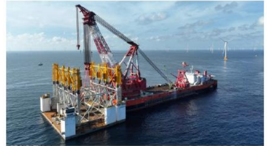
Installation in China of first 2GW VSC HVDC platform for offshore wind
