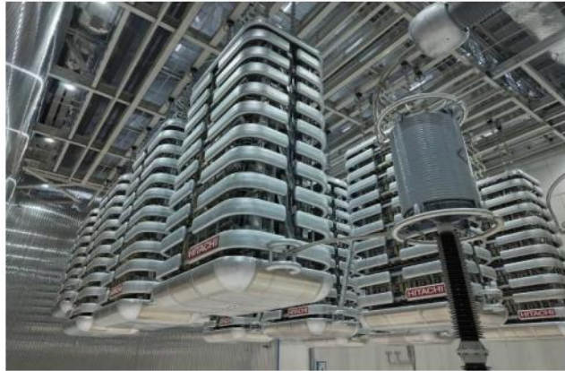
Commissioning of India's first VSC-HVDC to Mumbai city centre
