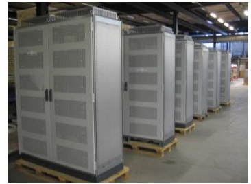
Caithness-Moray HVDC Replica Panels
